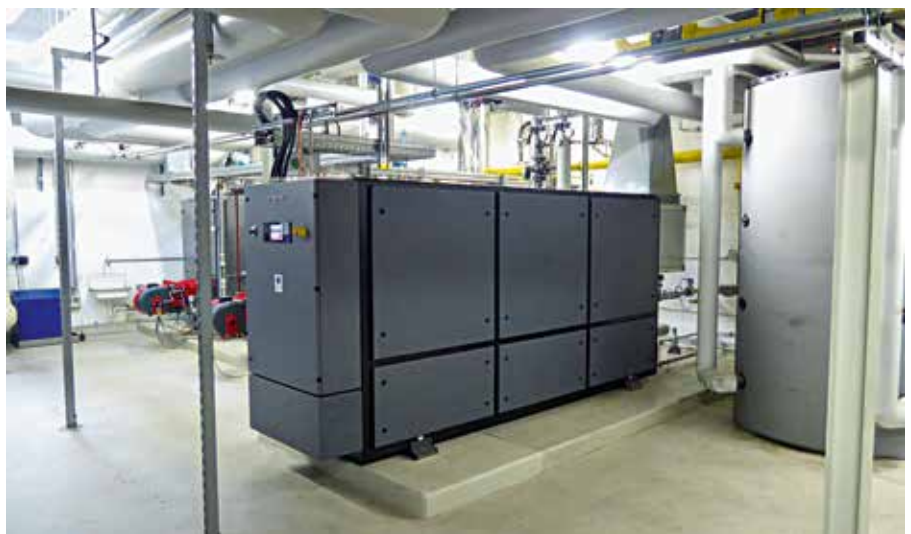
The cogeneration plant supplies the Hörmann site in Ichtershausen with energy.
