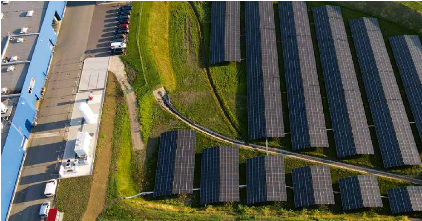
Supporting the process: The photovoltaic system supplies the PEM electrolyser with electricity, which in turn separates water into hydrogen and oxygen.
