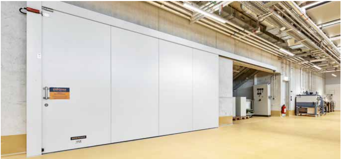
Protected fire compartment: The goods lift is located behind the sliding fire door.
