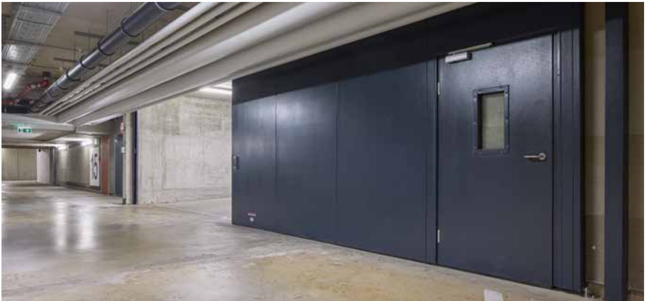
Standard doors and gates, such as this fire sliding door, are painted in a neutral anthracite finish.
